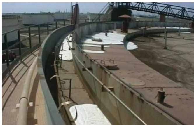
Too rich proportioning, meaning the foam solution cannot flow effectively to seal on a tank rim seal test (image courtesy of LaStFire)
